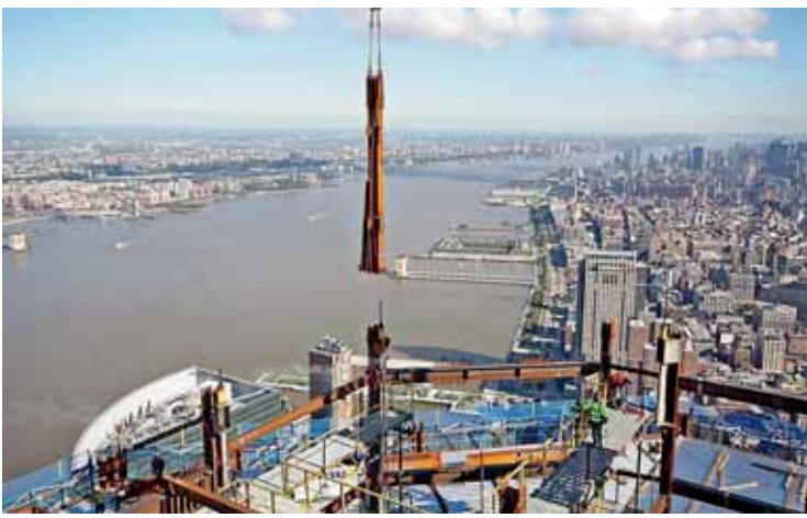
One of the steel members to the structure produced by the steel contractor MRP.
