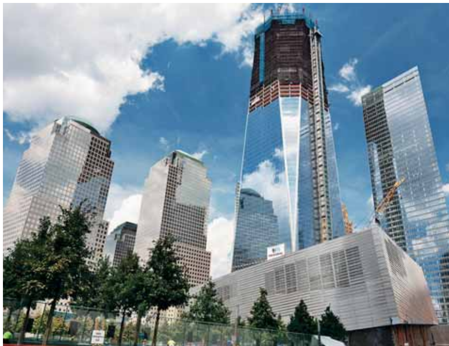
One World Trade Center, engineered by WSP Cantor Seinuk, will soon reach the top.
